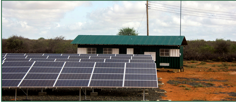
Biyamadhow Solar Project, Wajir South Constituency - Wajir County
